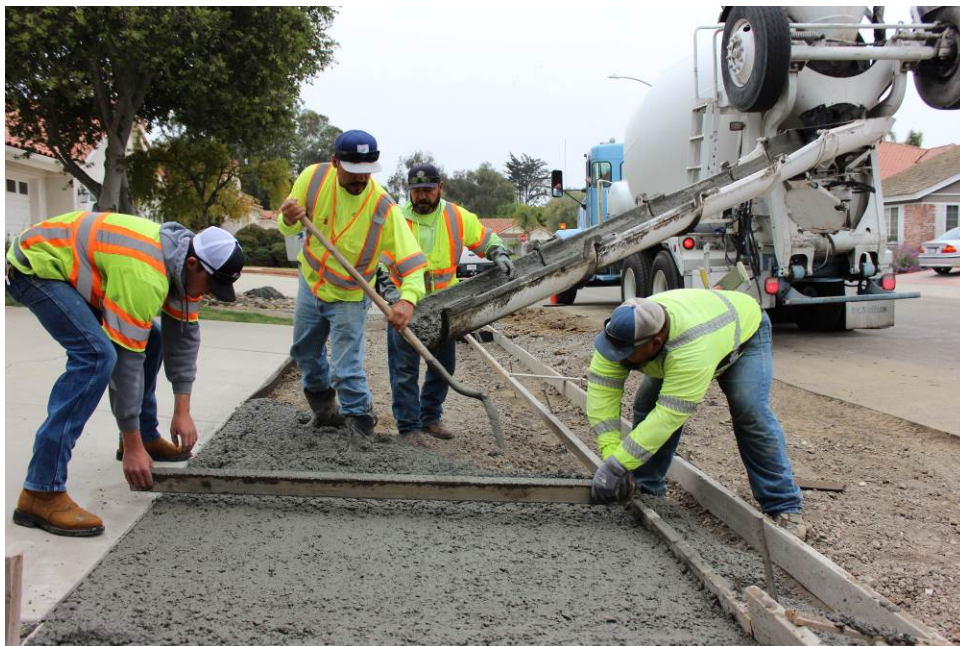
A replacement concrete curb, gutter, and sidewalk are poured and formed by the City's Public Works crew.
